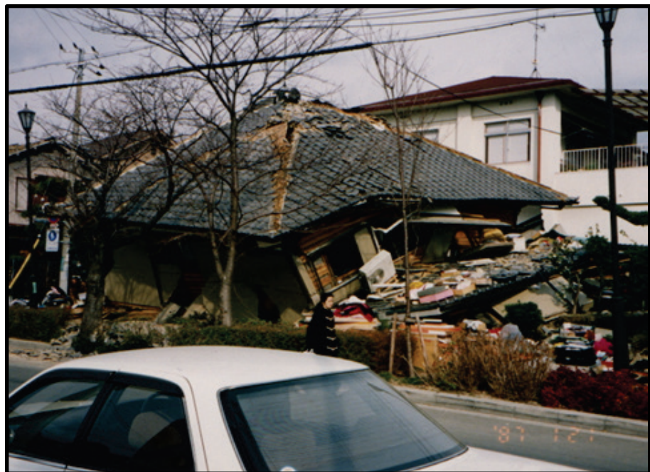
Figure 2-12 Partial first-story collapse of a two-story house with a heavy tile roof in Nishinomiya after the 1995 Kobe earthquake.
