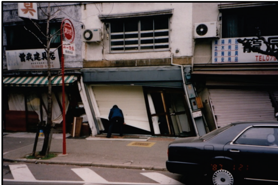
Figure 2-13 Severe leaning and incipient collapse of a two-story mixed-use building in Kobe City.
