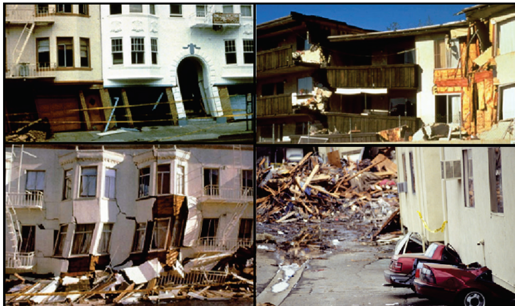
Figure 2-4 Collapse of soft-story wood light-frame multi-family dwellings in the 1987 Loma Prieta earthquake (left) and 1994 Northridge earthquake (right).
