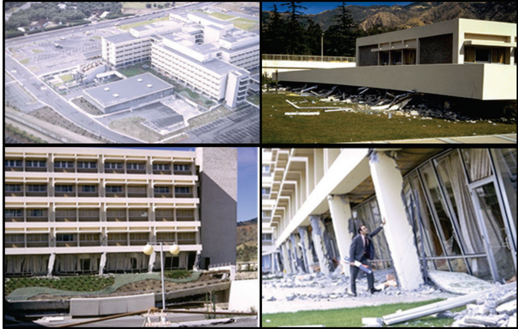
Figure 2-3 Collapse of the first floor of the two-story Community Mental Health Building (upper right) and severe damage to the five-story main building at the Olive View Hospital in the 1971 San Fernando earthquake.
