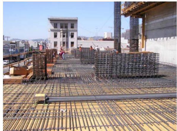
Figure 9-6 – Conflict between the location of collector reinforcing with a nonstructural component.
