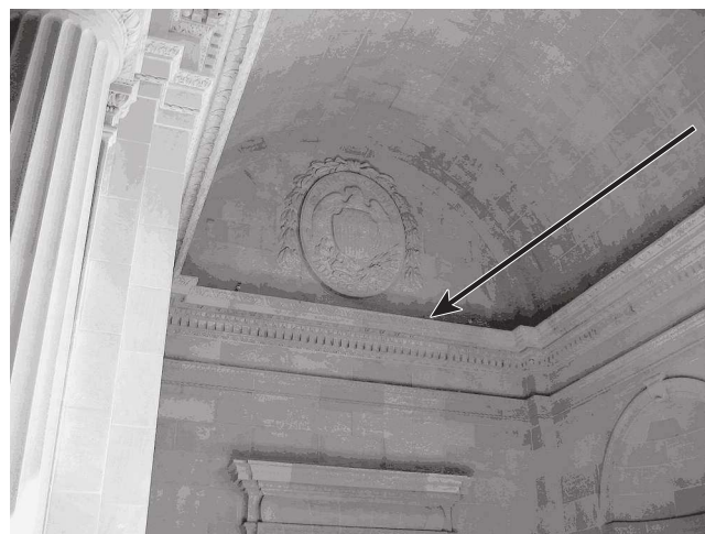
FIGURE F.3(c) Exposed Sprinkler Pipe.
